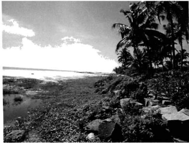
Fig. 47. Conspicuously noted are the remnants of the old collapsed seawall over which thick vegetation has thrived. Further seaward is the beach of uniformly sorted sands. (Punnapra)
