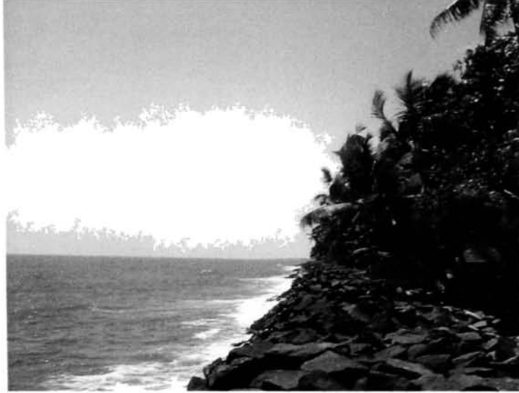
Fig. 19. The seaward view at Manasserry facing north. Note the height of the seawall around 2m just adequate to face the wrath of the monsoon breakers.
