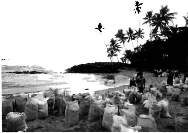
Fig. 28. A better view of the filled-up sand bags ready for placement along the shoreline at Pallithodu.
