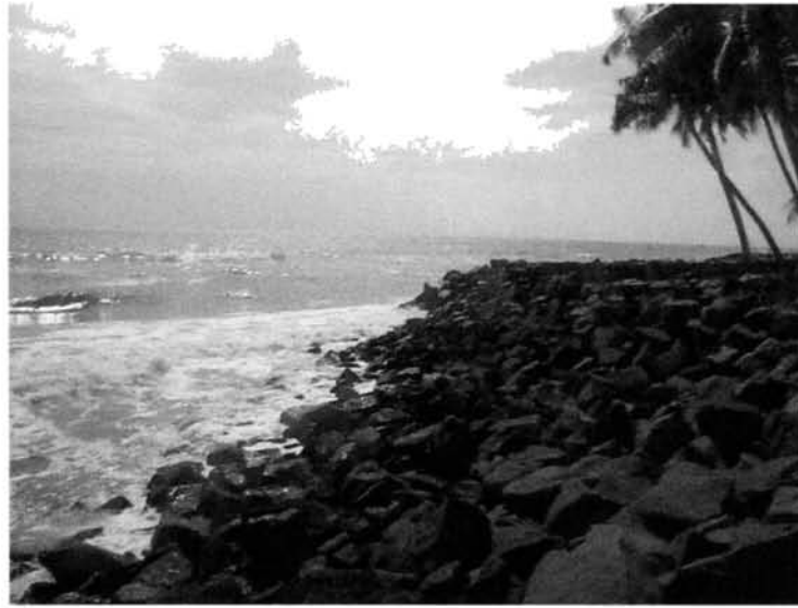
Fig. 23. The broad upper plateau of the seawall at Chellanam which shows early indications of frontal collapse.
