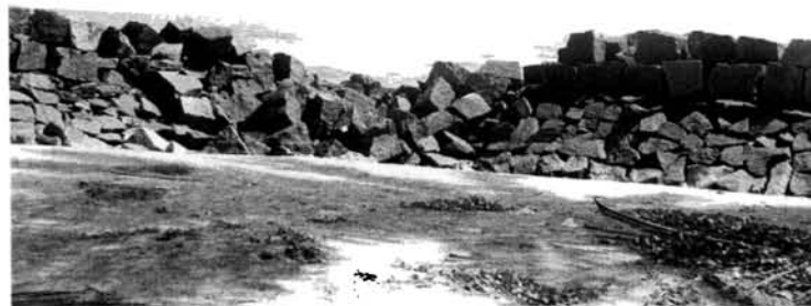
Fig. 21. Towards the seafront a collapse of a seawall permits run up of waves onto the backshore. Left alone the chances of breach of the seawall and subsequently extensive damage to either sides of the wall and resultant erosion could be a serious concern. (Kannamaly)
