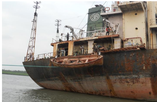
Fig. 3.10 Removal of Rescue Boat
