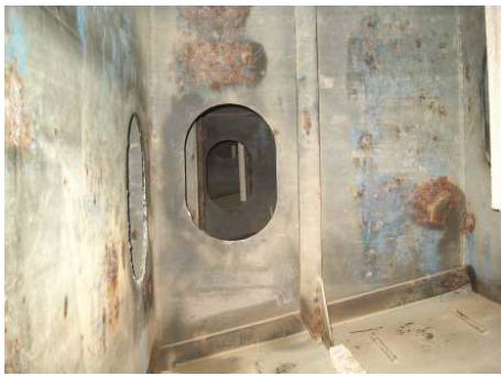
Fig 2.3 (c) Minor spot rusting (5% - 20% light rust)
