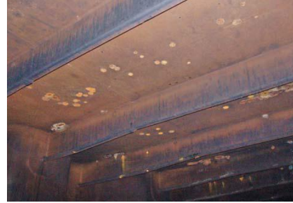
Fig 2.4 (b) Shallow pits < 5% Depth < 1/3 of original thickness
