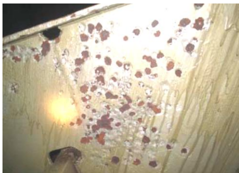
Fig 2.4 (e) Deep pits < 15% Depth > 1/3 of original thickness
