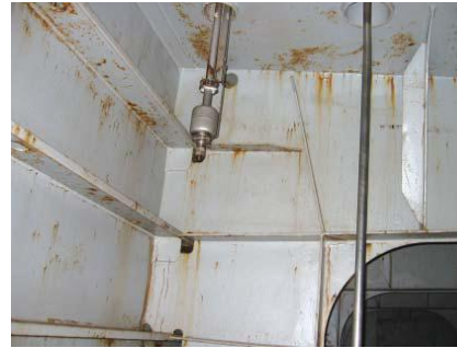
Fig 2.2 (b) Minor spot rusting
