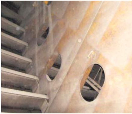
Fig 2.3 (a) No rusting
