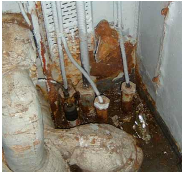
c) Corrosion of internal structure
