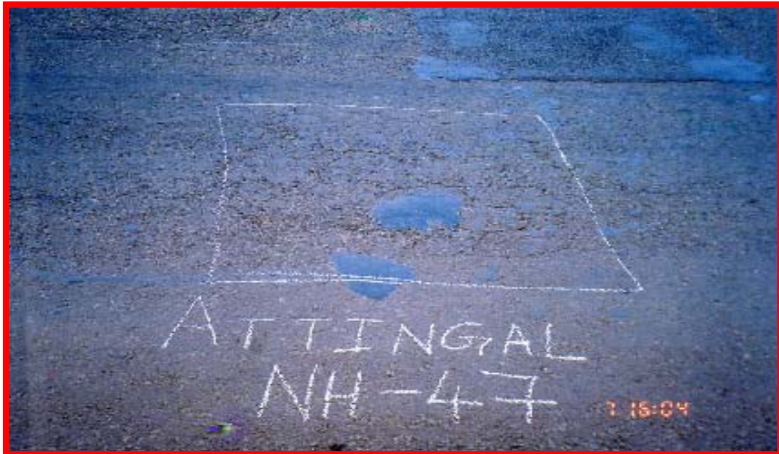
Fig. 3.4 Cracks with patching
