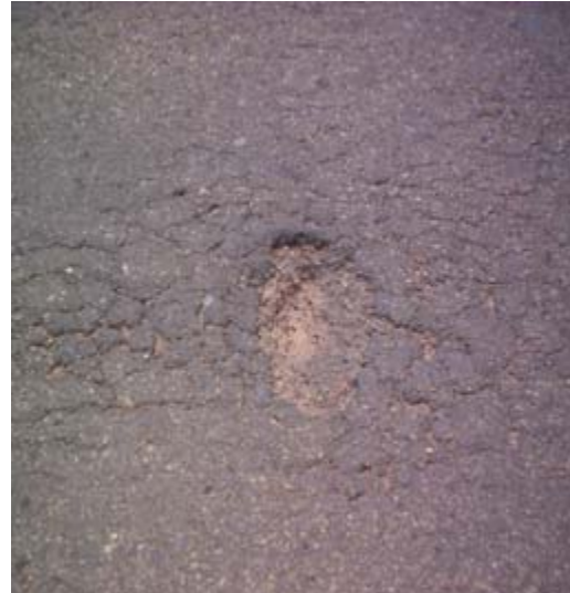
Fig. 3.6 Pothole and Alligator Cracks
