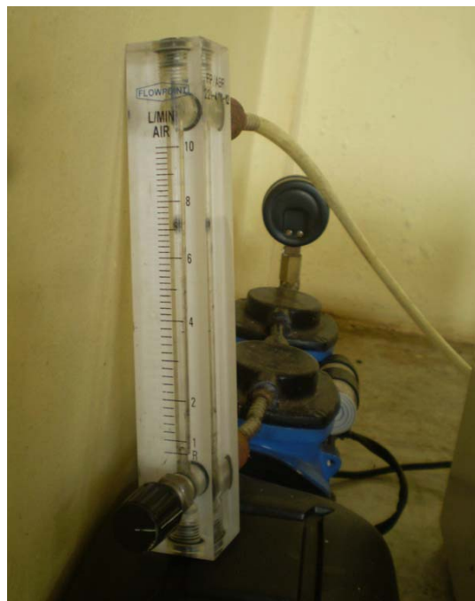
Fig. 3.4 Air compressor with flow meter
