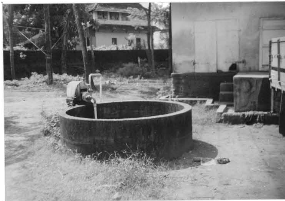
PHOTOGRAPH - 6 TYPICAL COASTAL WELL FITTED WITH PUMPSET
