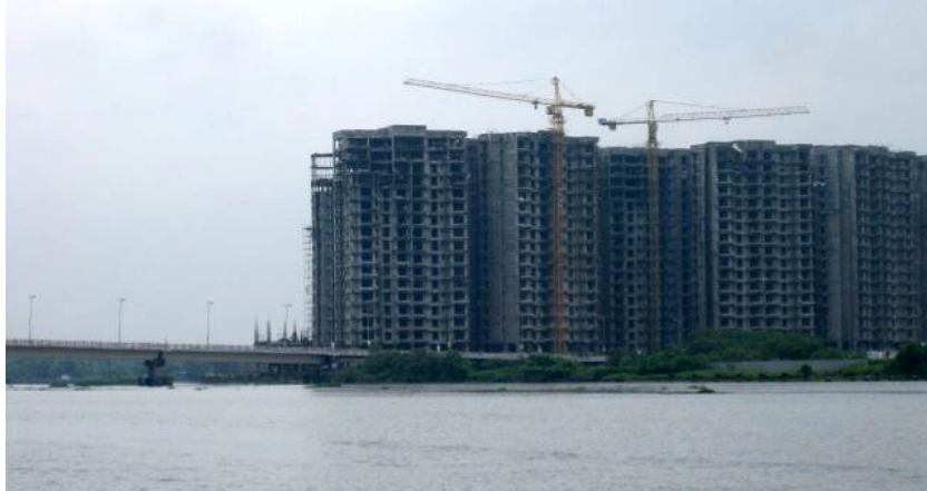
Plate 2.8 Station 4- Marine science Jetty Construction of apartments near Marine Drive during the sampling period.
