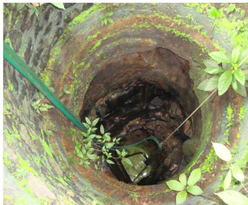
Fig.4: Dug cum Bore well
