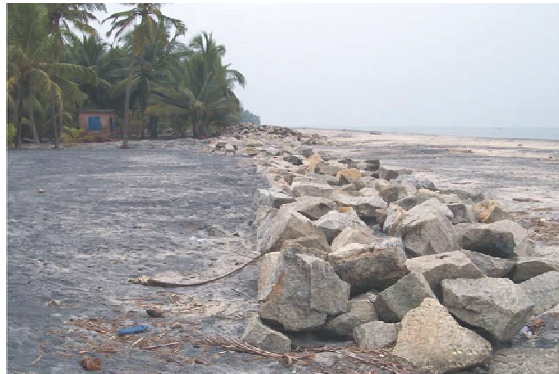
Figure 1.10: The sea wall sinks and gives in to the persistent sorties of the waves and toe erosion. A view of Alappad beach
