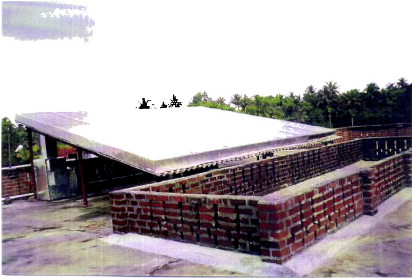
Fig. 4.4 A 46 m 2 solar air heater installed in the food processing industry
