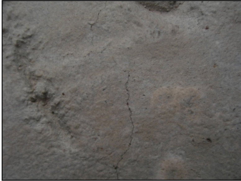
Figure 6.72 Typical major crack in CC heated to 600°C-closer view.
