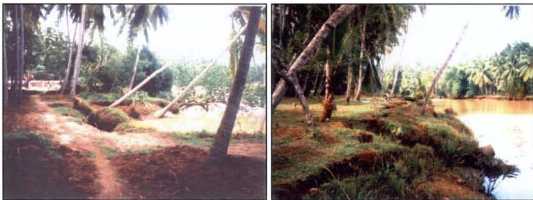
Plate 7.2 A close-up of the river bank in the lowlands showing bank failure incidences due to river bed lowering and indiscriminate sand mining
