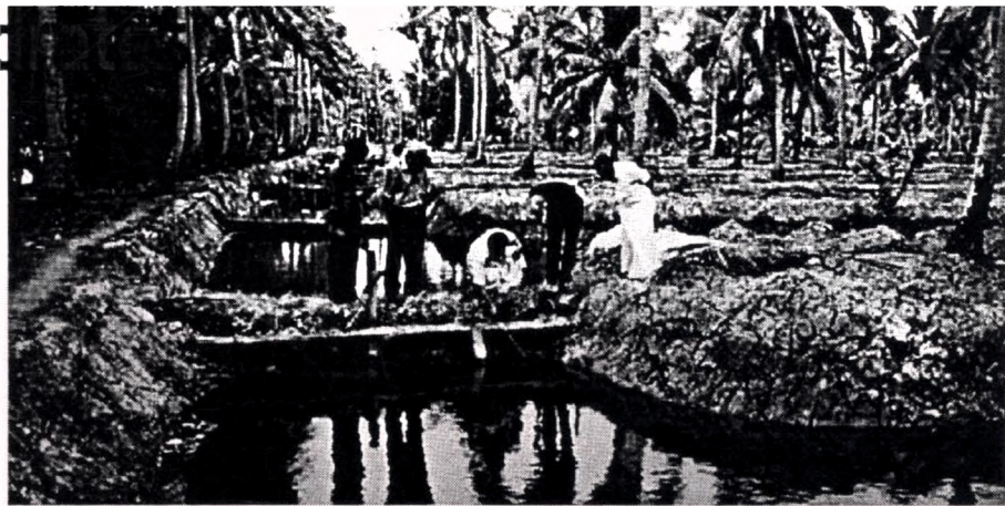
Small dams were built in water channels to make the 250-m 2 test ponds.
